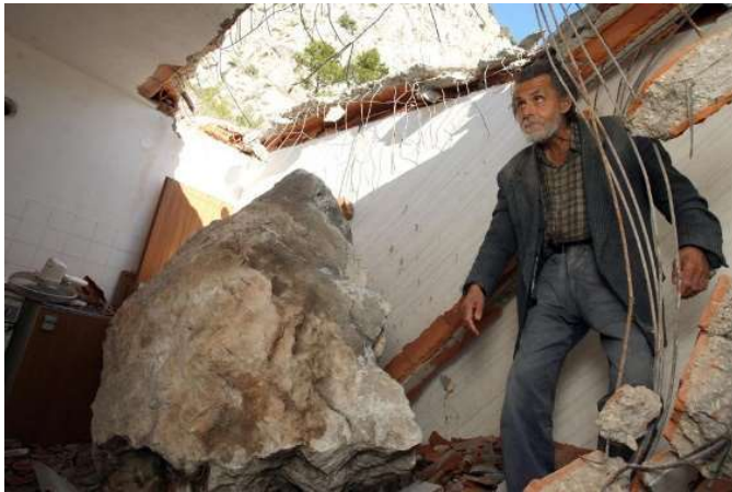
Figure 2 Fallen rock block came through the roof in the house in January 2012 ( www.24sata.hr ).
