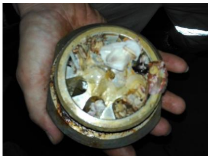
Figure 6 - Contaminated nozzle (Wärtsila Moss scrubber unit)
