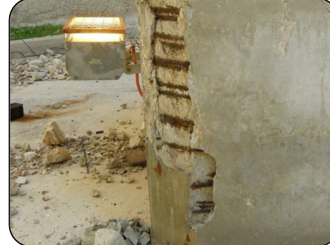
Maslenica: Reinforcement corrosion on column S10
