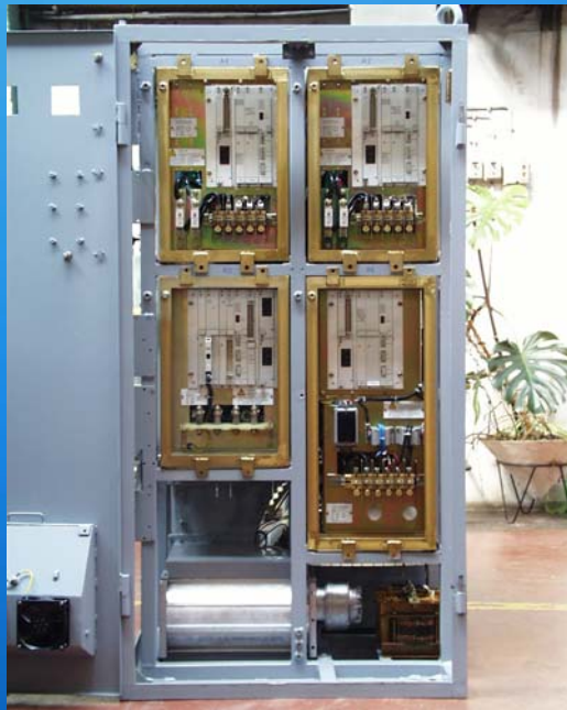
Converter with 5 output inverters plus battery charges
