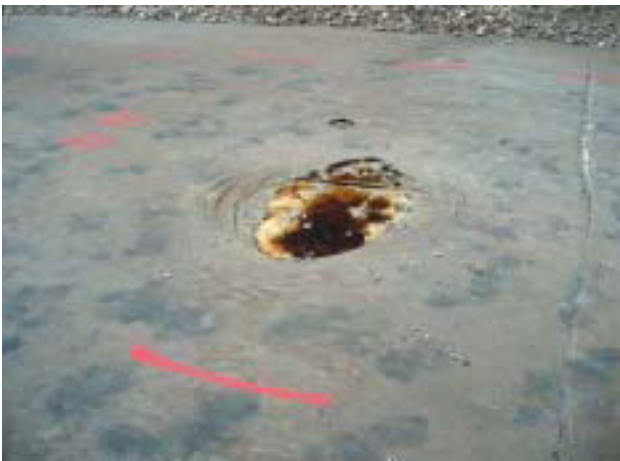
Figure 2. Smaller geomembrane rupture in damaged zone
