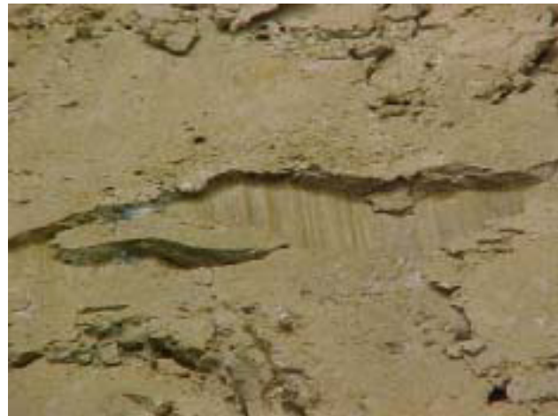
Figure 3. Slippage of softer clay layer over firm clay base
