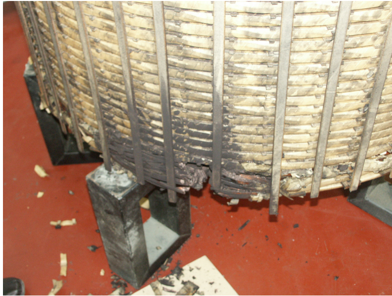
Figure 7. Turn-to-turn fault at the end of the common winding of the Autotransformer Tr3
