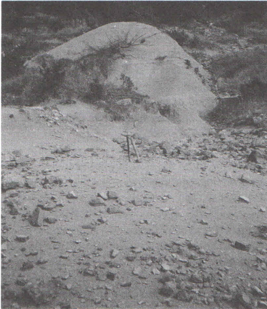
Figure 1B. Effect of erosion of slope made of flyschin the region of Istria.
