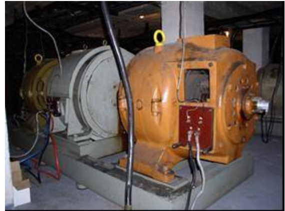
Fig. 8. Synchronous generator with prime mover DC motor
