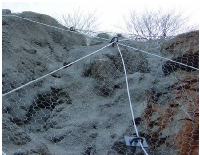
Figure 6. Slope protection with galvanized meshes reinforced with rockbolts and steel wire ropes
