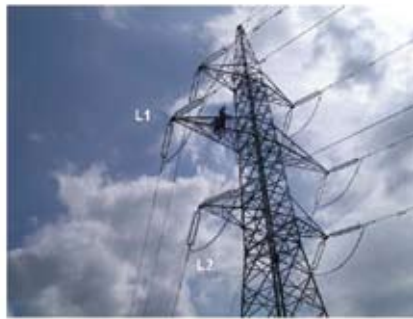
Slika 10 — Raspored vodiča na 49-om stupu Figure 10 — Arrangement of the conductors on the 49 th tower
