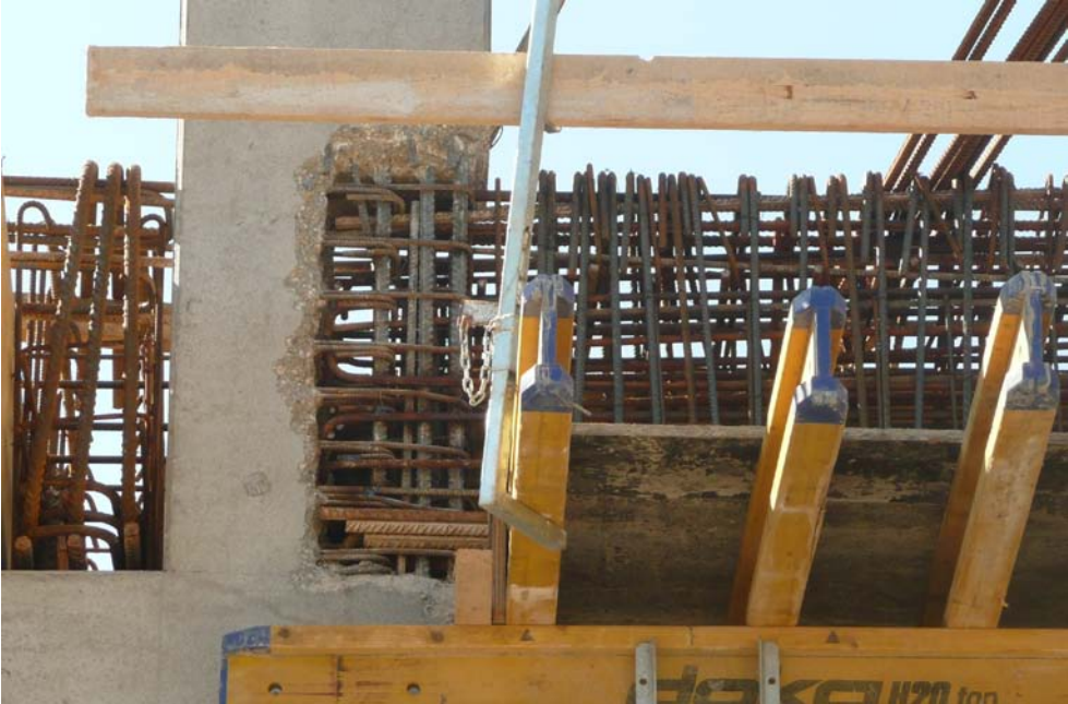
Figure 3: Due to poorly perfected project documentation mounting of monolith beam was impossible without additional processing of the precast element
