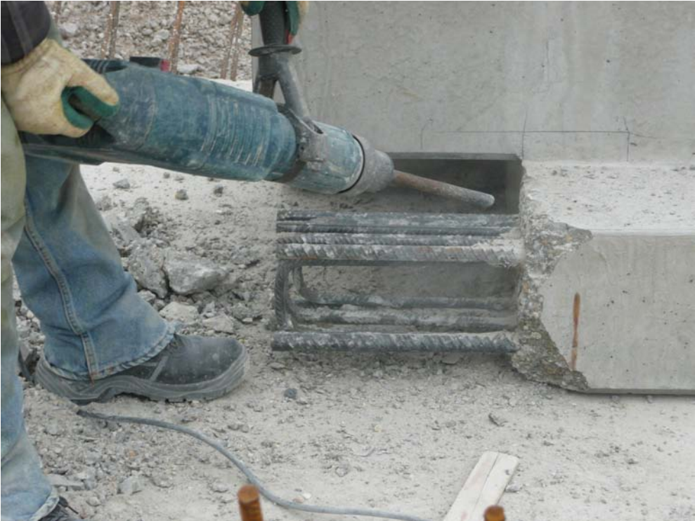
Figure 4: Poorly perfected project documentation resulted with a need to additionally process the precast element
