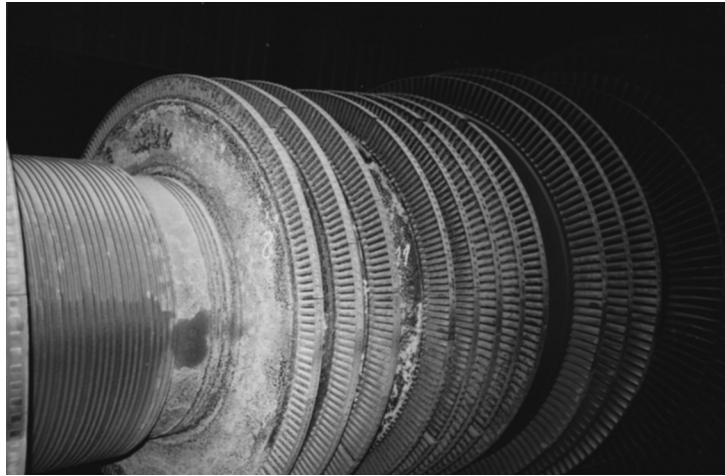
Figure 4. Corrosion and deposits of turbine rotor
