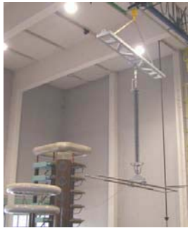
Fig. 4. C: 220 kV single suspension polymer insulator string
