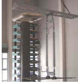
Fig. 3. B: 110 kV double suspension polymer insulator string
