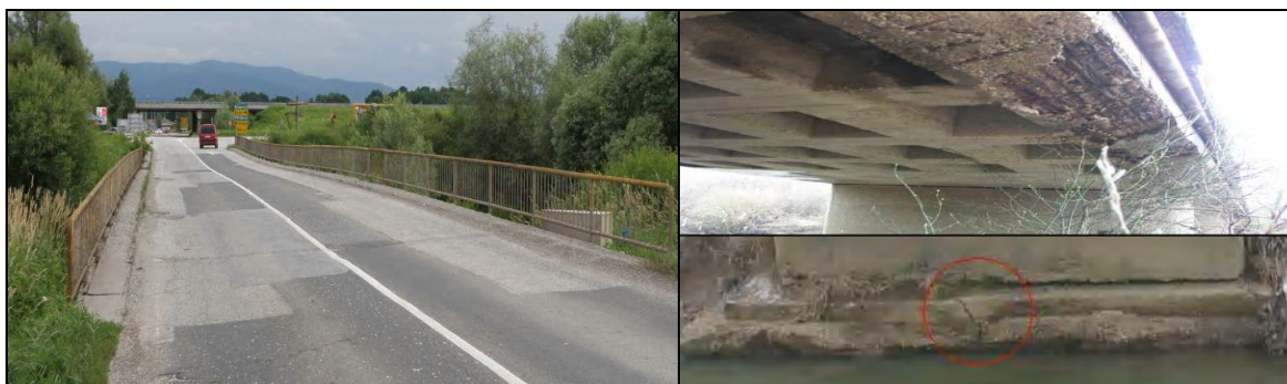
Fig. 2 View of the old bridge Mokrice with details of damages in edge beams and pier foundation
