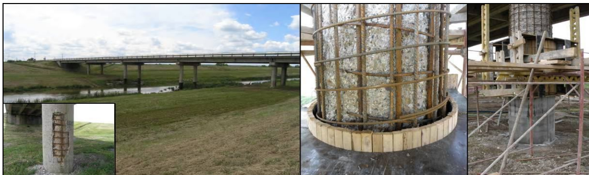
Fig. 4 The Vukovina bridge with details of column damages and strengthening by steel
