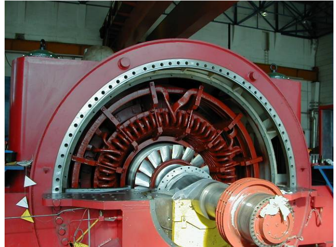
Fig. 1. Turbogenerator 247 MVA, 13.8 kV, \cos\phi_n=0.85 , 3000 \text{min}^{-1}
