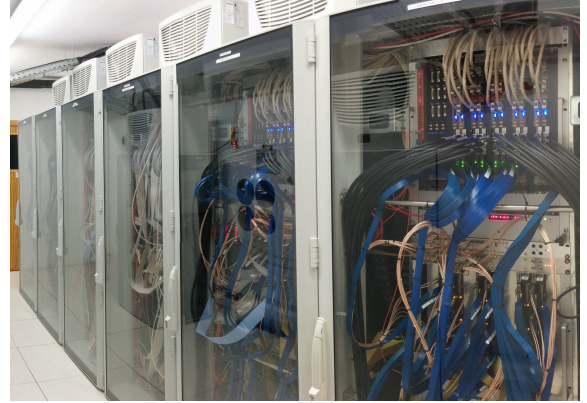
Figure 7: View of the electronics room of the MAGIC telescopes. The six closed racks can be seen. They are placed on a technical raised floor (20 cm height) allowing for better cable routing.
