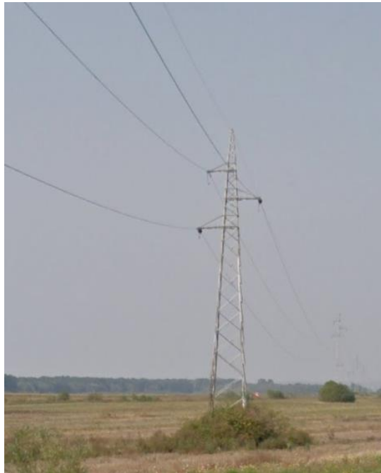
35 kV overhead line with steel lattice towers and a single shield wire
